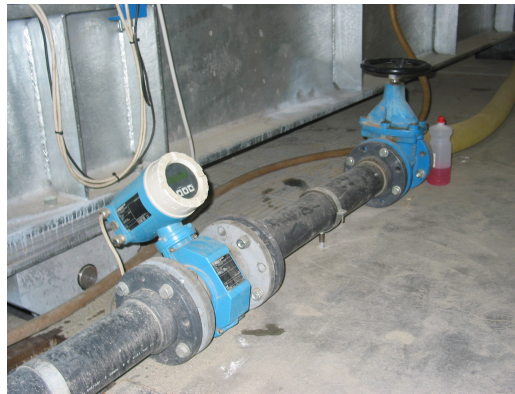
Figure 4.4: The electromagnetic flowmeter.
